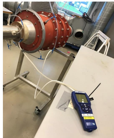
Elliptic nozzle used for the air flow measurement
