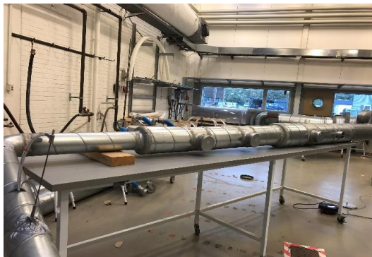
Duct system with pitot tube for the static pressure before inlet
